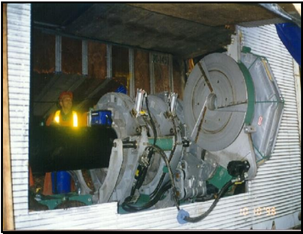
450 mm dia. fusion welding machine for the HDPE pipe was used in a special shelter to avoid driving rain and wind (typical during winter months in Ucluelet) during the heat fusion welding process.
